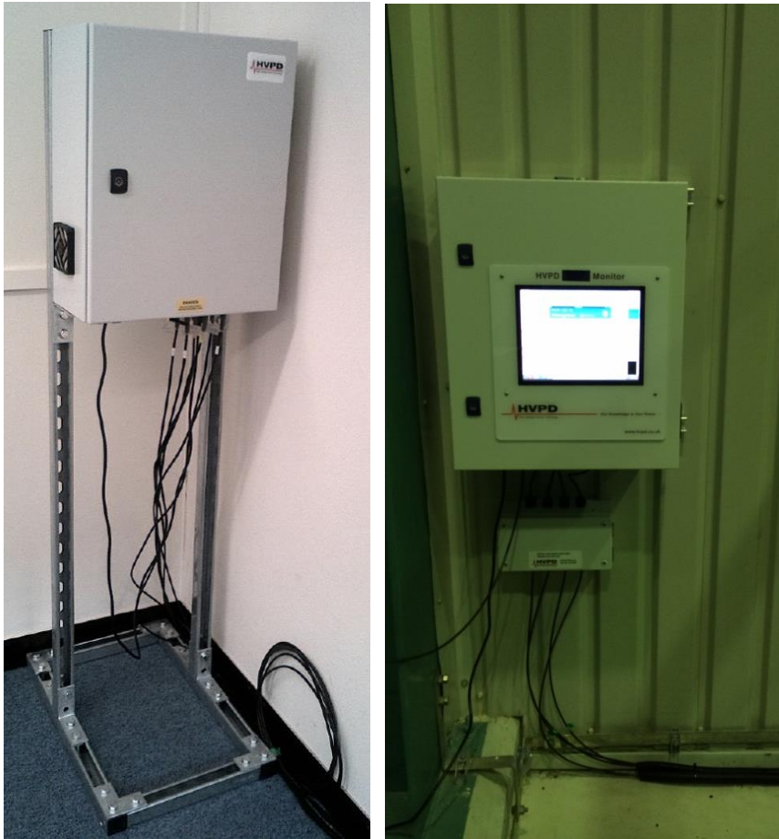
Photos of installed HVDC OLPD Alpha monitor systems at Alstom Grid HVDC Cable Ageing Facility and a HVDC interconnector
